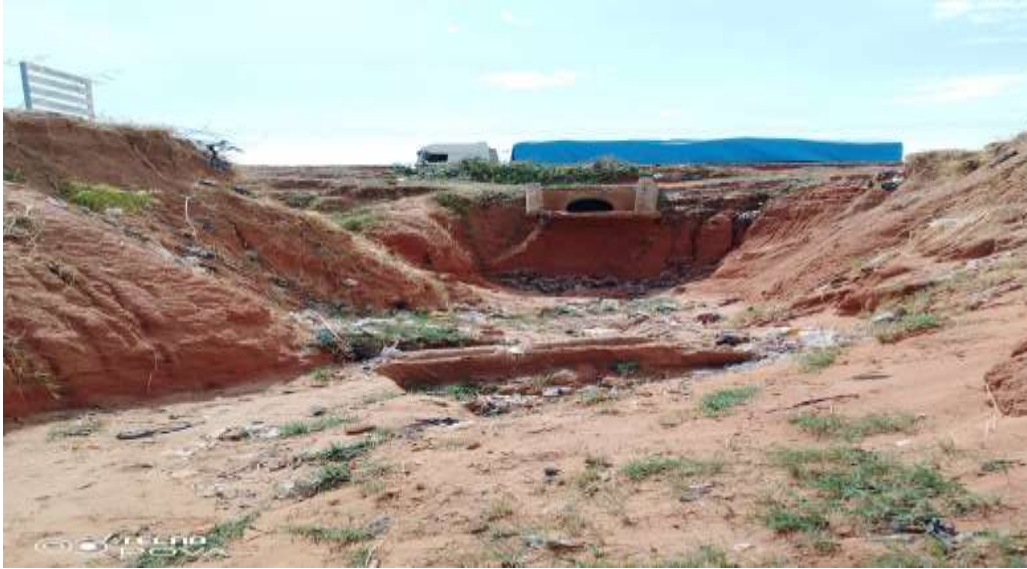
Plate 1: Bye-pass road in Gombe threatened by head ward retreat of gully erosion in the area
