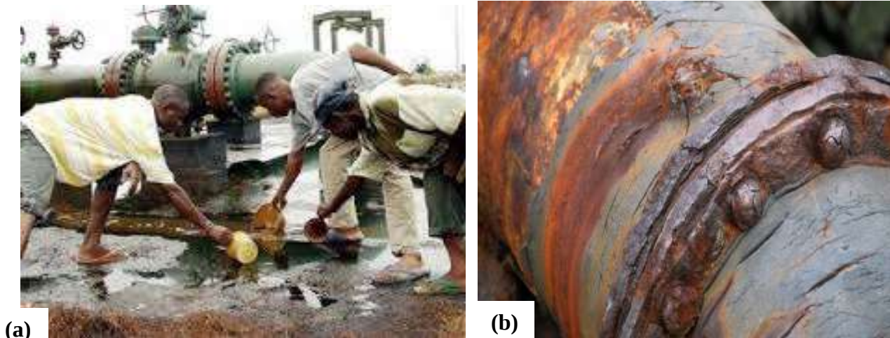
Figure 5: Pipeline corrosion (b) with its easiness towards pipeline vandalization (a)
