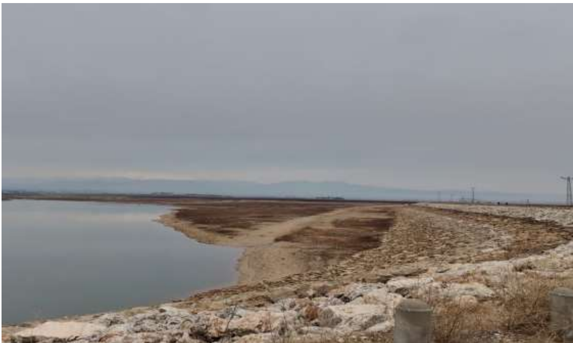
Figure 3. Çamgazi Dam water level and previous water-level marks on the embankment (Z.Kılıç)
