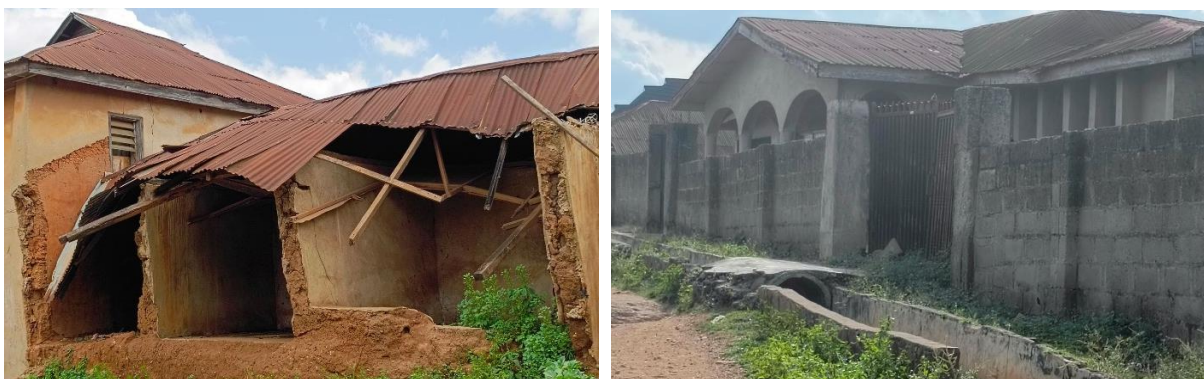
Figure 7: Decrepit buildings in Ibule-Soro and home requiring major facelift in Oba-Ile
