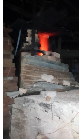
Fig. 16: Flame coming out of the chimney
